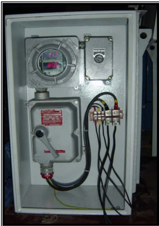
OIL TYPE UNIT TRANSFORMER RECTIFIER
